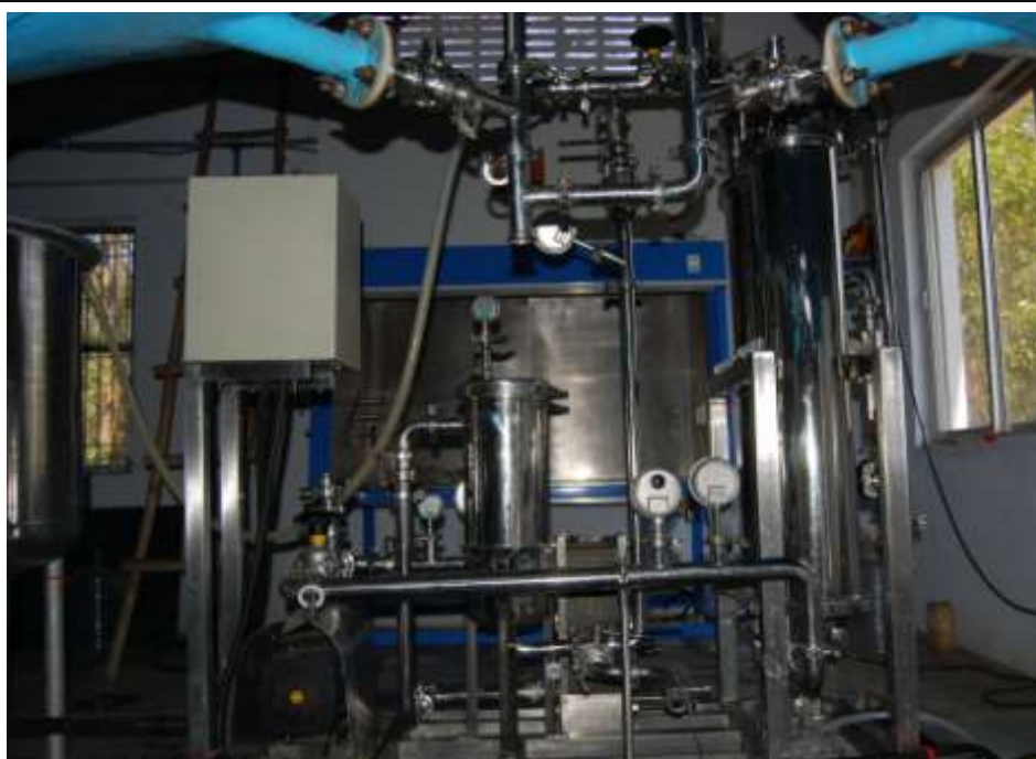
Neera Filtration Plant in CFC of Cluster
